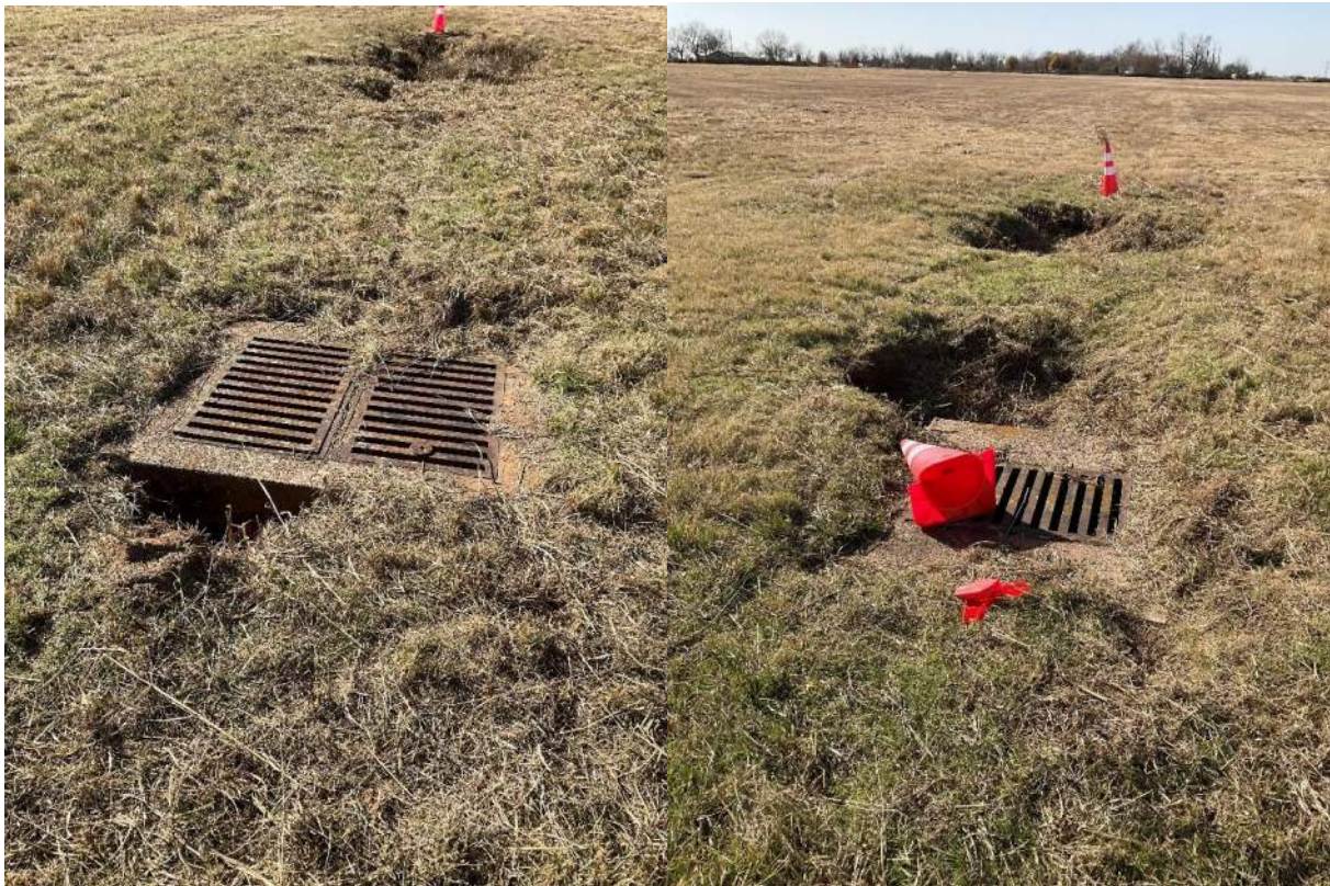
Figure 4: Erosion around inlets and sink holes south of Taxiway F
