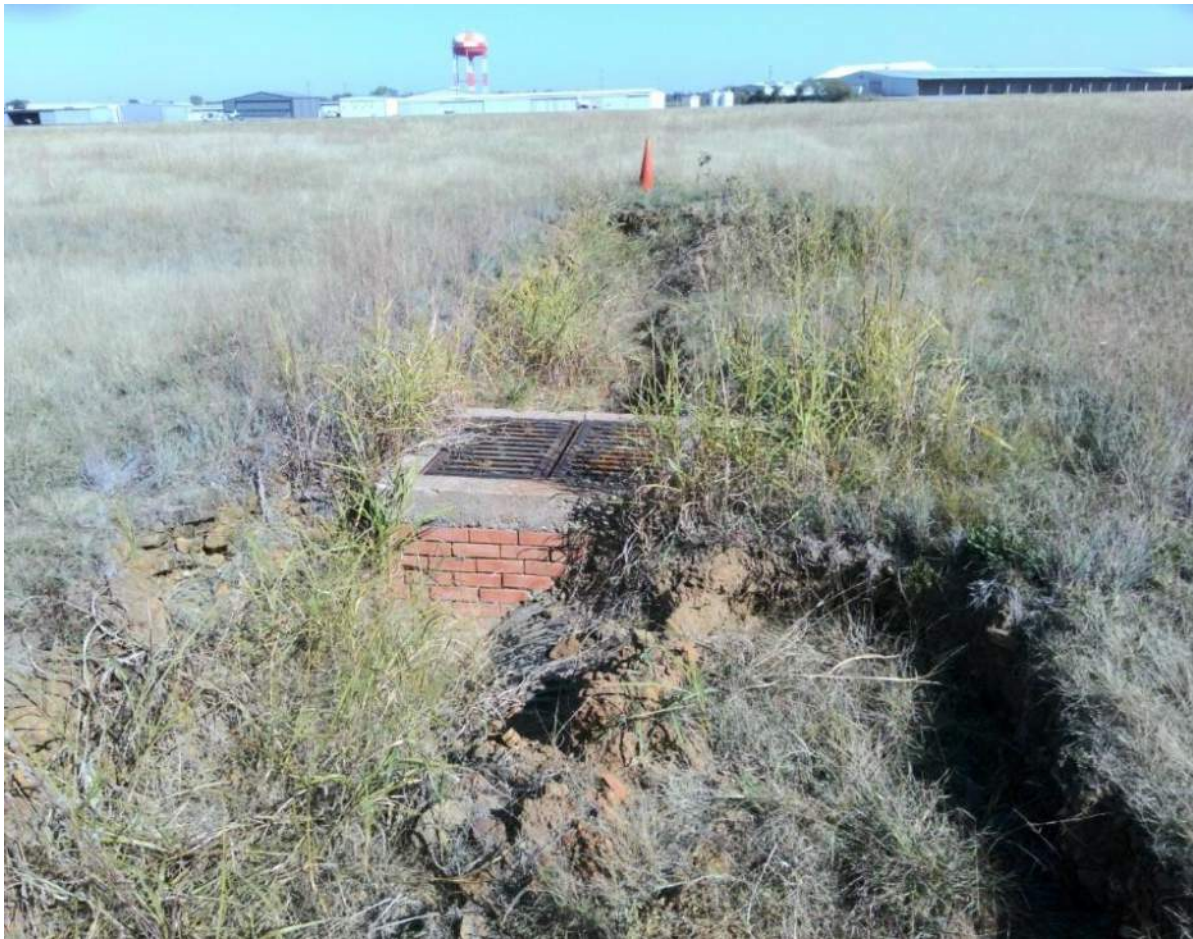
Figure 3-15. Erosion Near Taxiway F
