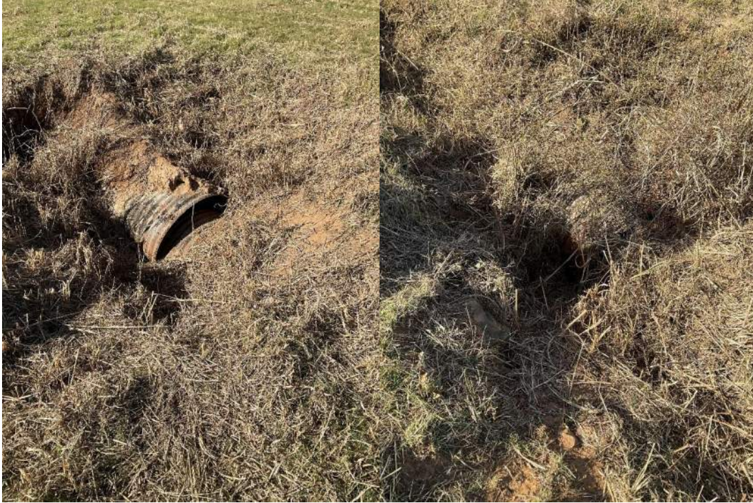
Figure 3: Exposed pipes south of Taxiway F
