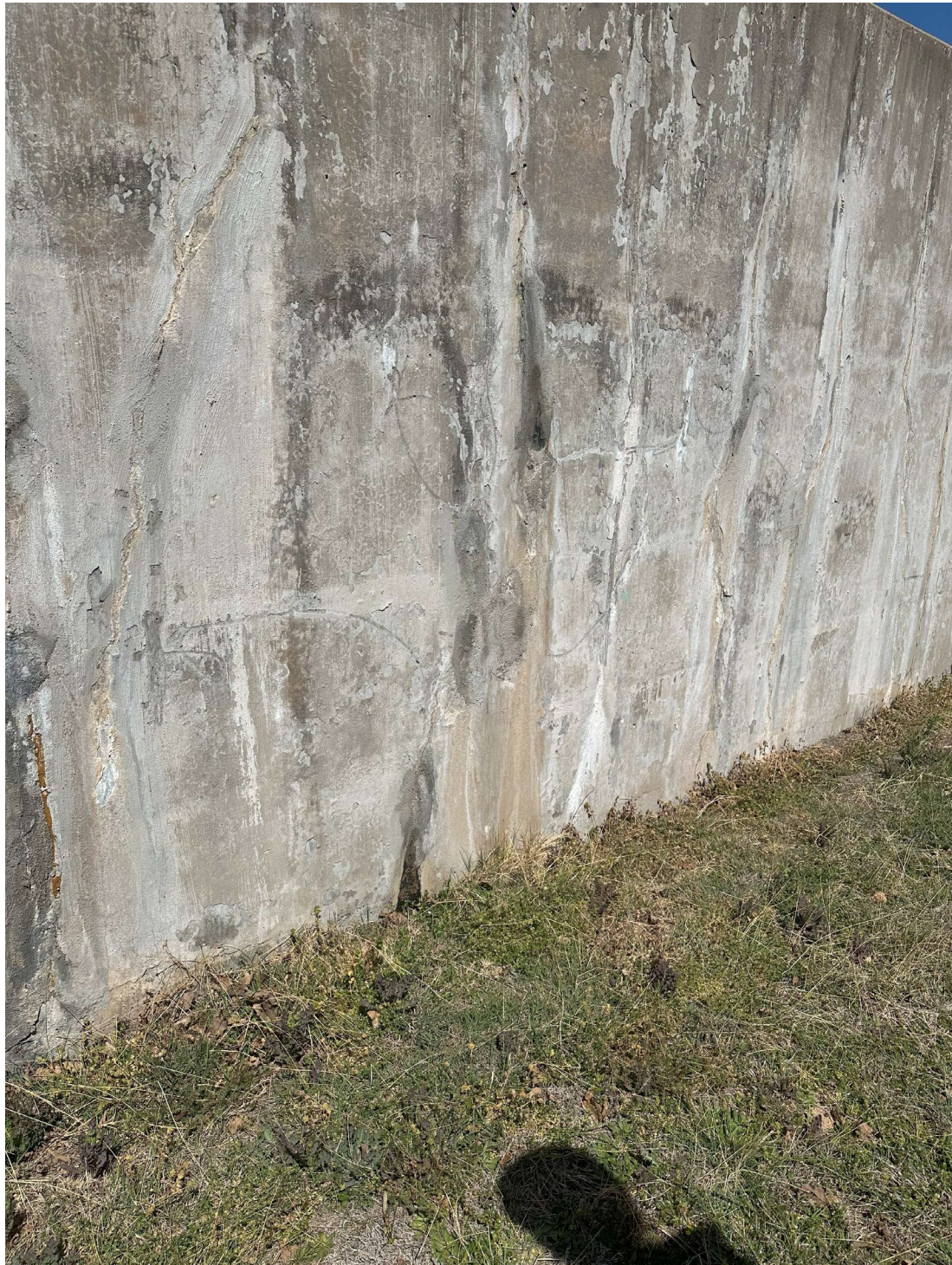
Figure 3-7. Cracks on Exterior Walls
