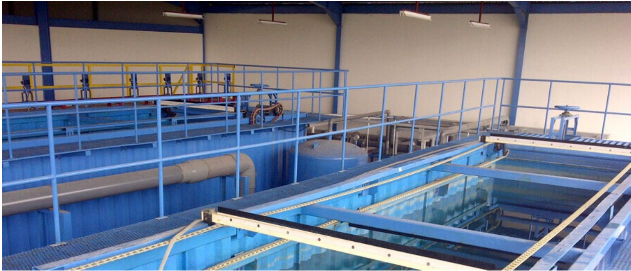
Figure 4-3. Dissolved Air Flotation Tank
