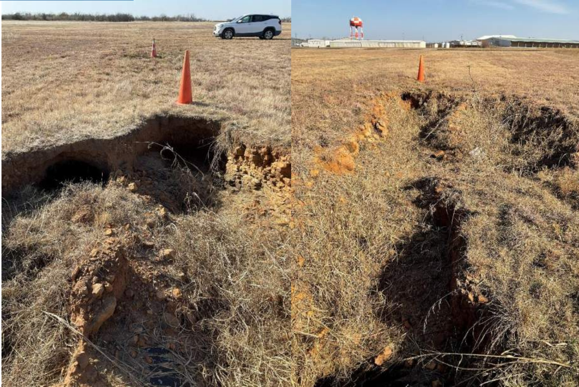
Figure 1: Collapsed areas around drainage pipe west of Runway 13-31
