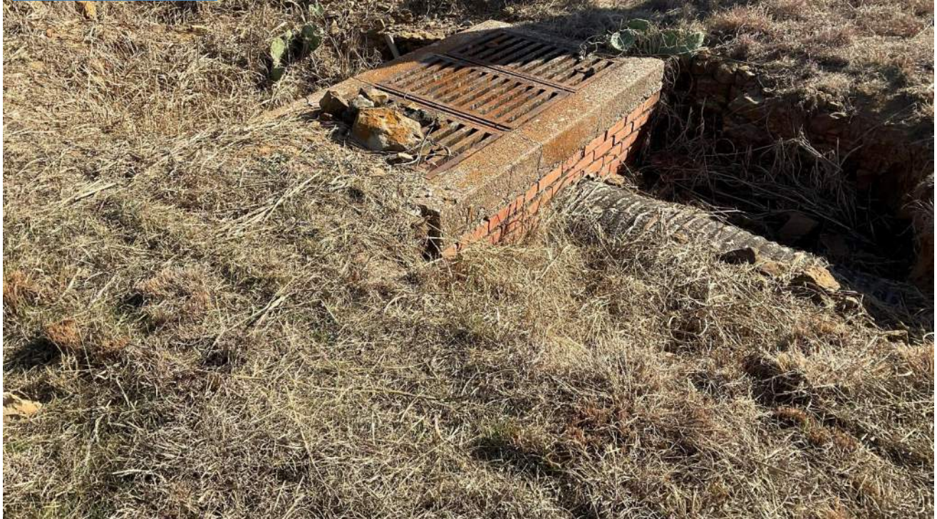
Figure 5: Erosion and exposed pipe around inlet south of Taxiway F
